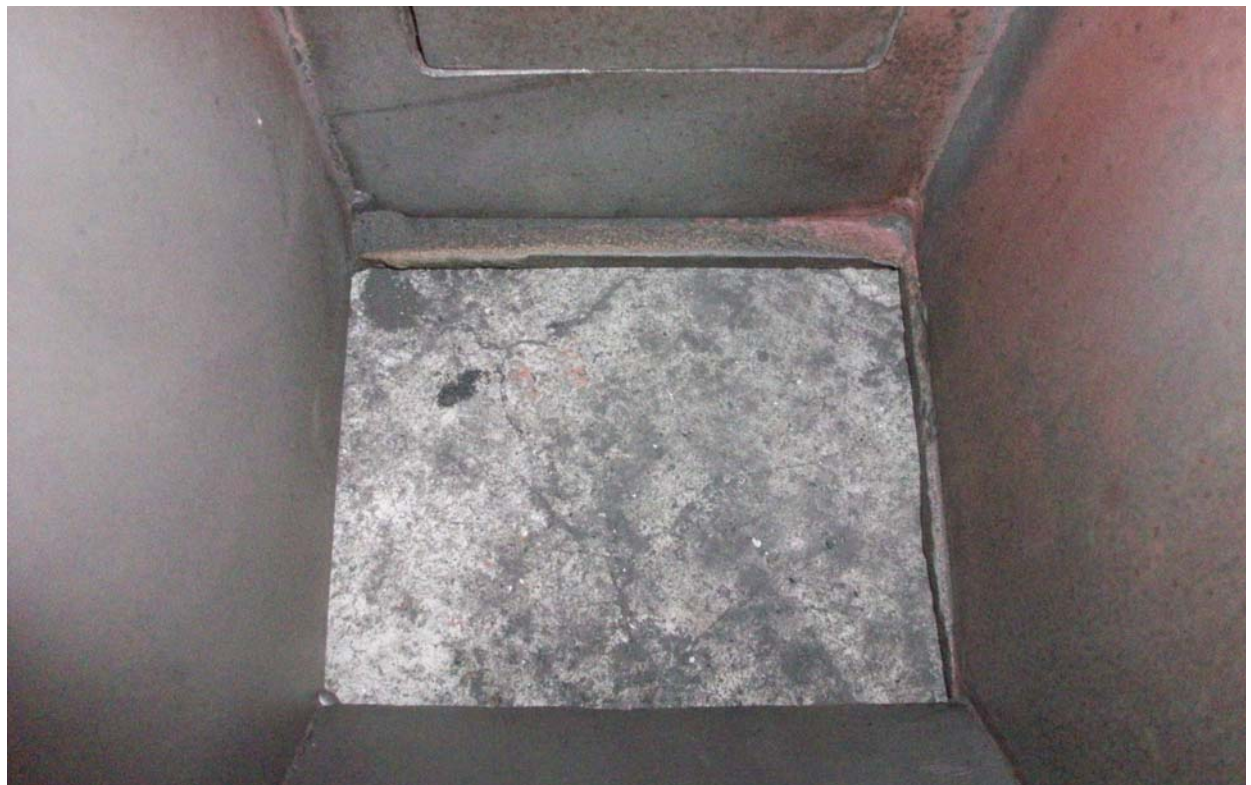
Photo 14: Mismatch in flange setting is seen here. Such protrusions can act as support for wet coal dust.
