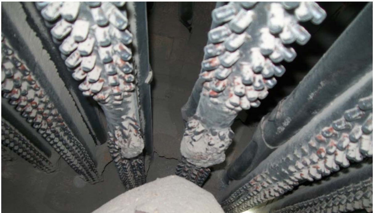
Photo 2 & 3: It is seen the protective coating by phoscast is seen dislodged. Right above the fuel nozzles only the erosion is seen. This can happen due to high fuel line air flow.
