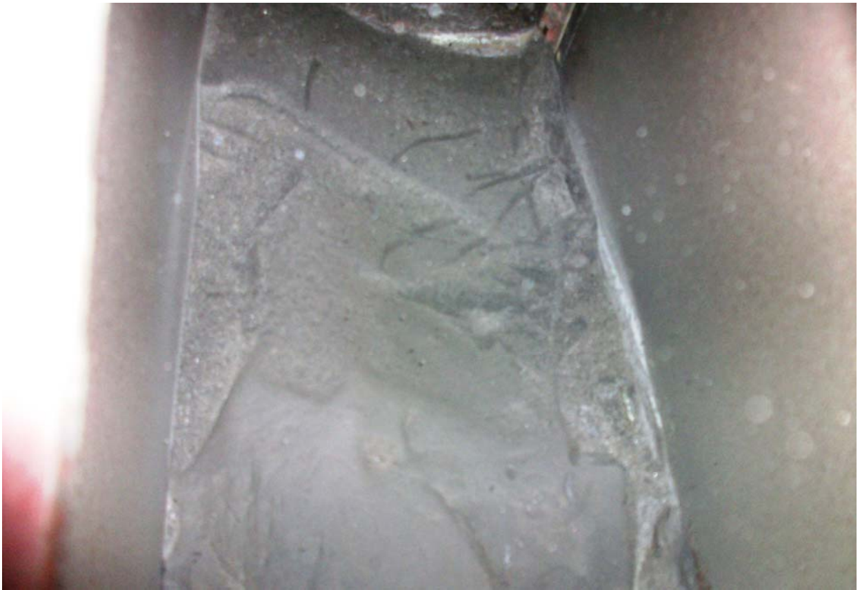
Photo 10: Coal dust seen to build up on the sloped plate of mixing nozzle inlet chute. The coating was seen to be quite strong. Incidentally all the old mixing nozzle inlet chutes were seen to be like this.
