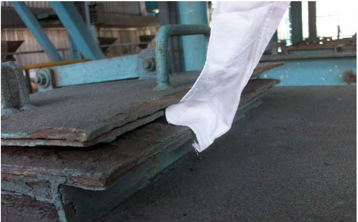
Photo 4: The suction effect seen at feeder in boiler no 1, where the mixing nozzles were replaced by a lower diameter throat. The feeder area was now seen to be free of dust.
