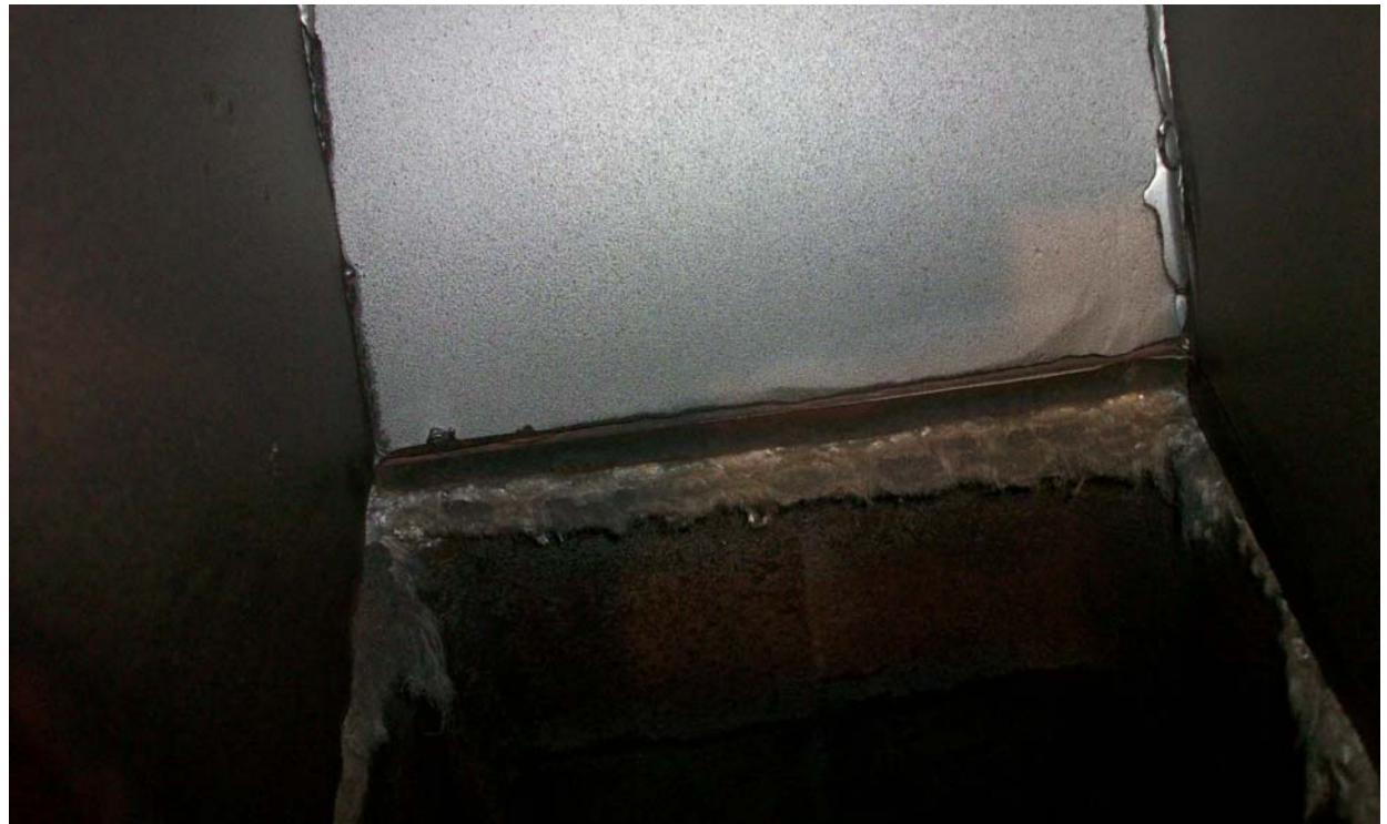
Photo 9: The asbestos pad provided above the mixing nozzle was seen to be projecting in to the coal path. Wet coal dust could get a support over this and eventually lead to arching.
