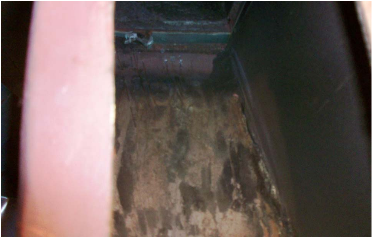
Photo 11: The same chute plate after cleaning is seen here. The dust is seen to have built up on the weldment of liner plate.
