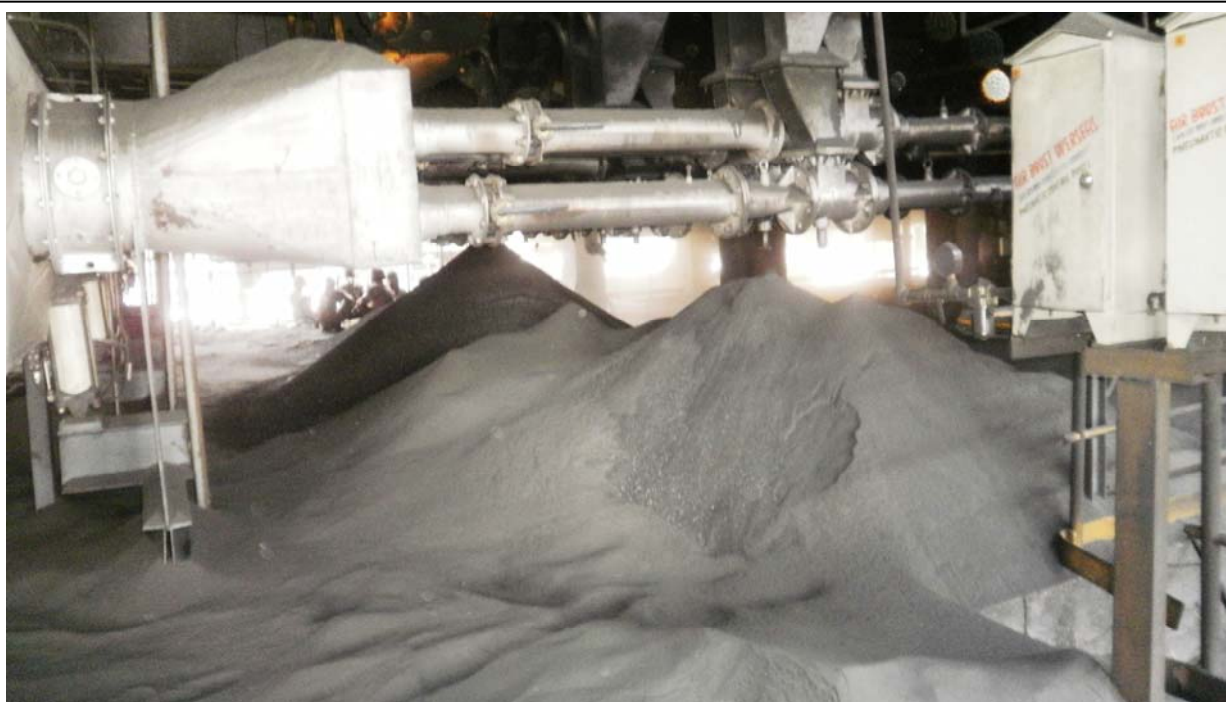
Photo 1: The dust nuisance experienced at PA lines. The lines get choked often and then dechoking led to coal accumulations at feeder floor.
