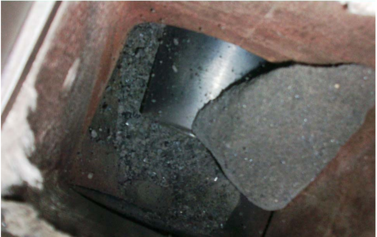
Photo 15: In one of the mixing nozzles, it was found that the coal lump was lying above throat. The Coal dust could build up from here.
